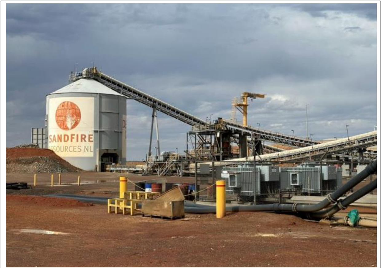
Figure 3: DeGrussa Process Plant
